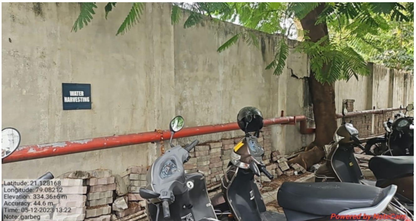
Water Harvesting Pipes Connection
