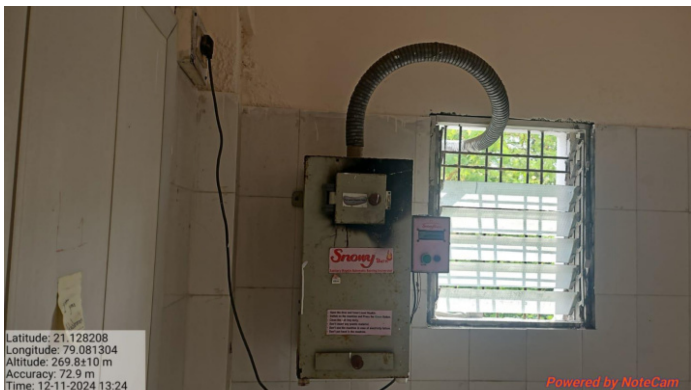
Incinerator in girl's washroom
