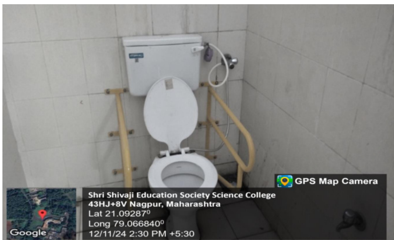
Washroom for Divyangjan
