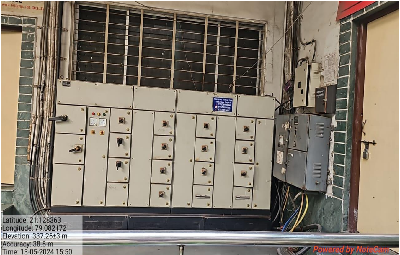
Solar converter / Generator / Electric distribution unit
