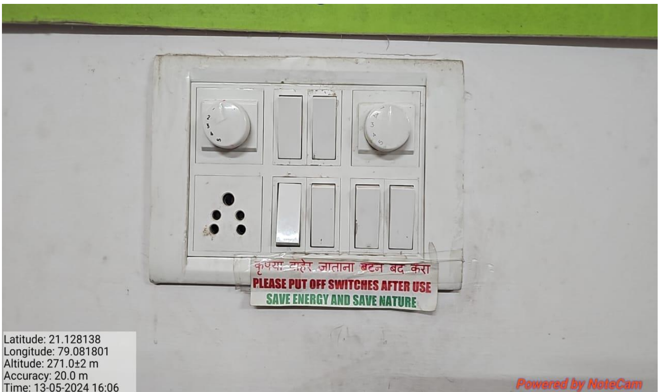
Signage for Energy Saving
