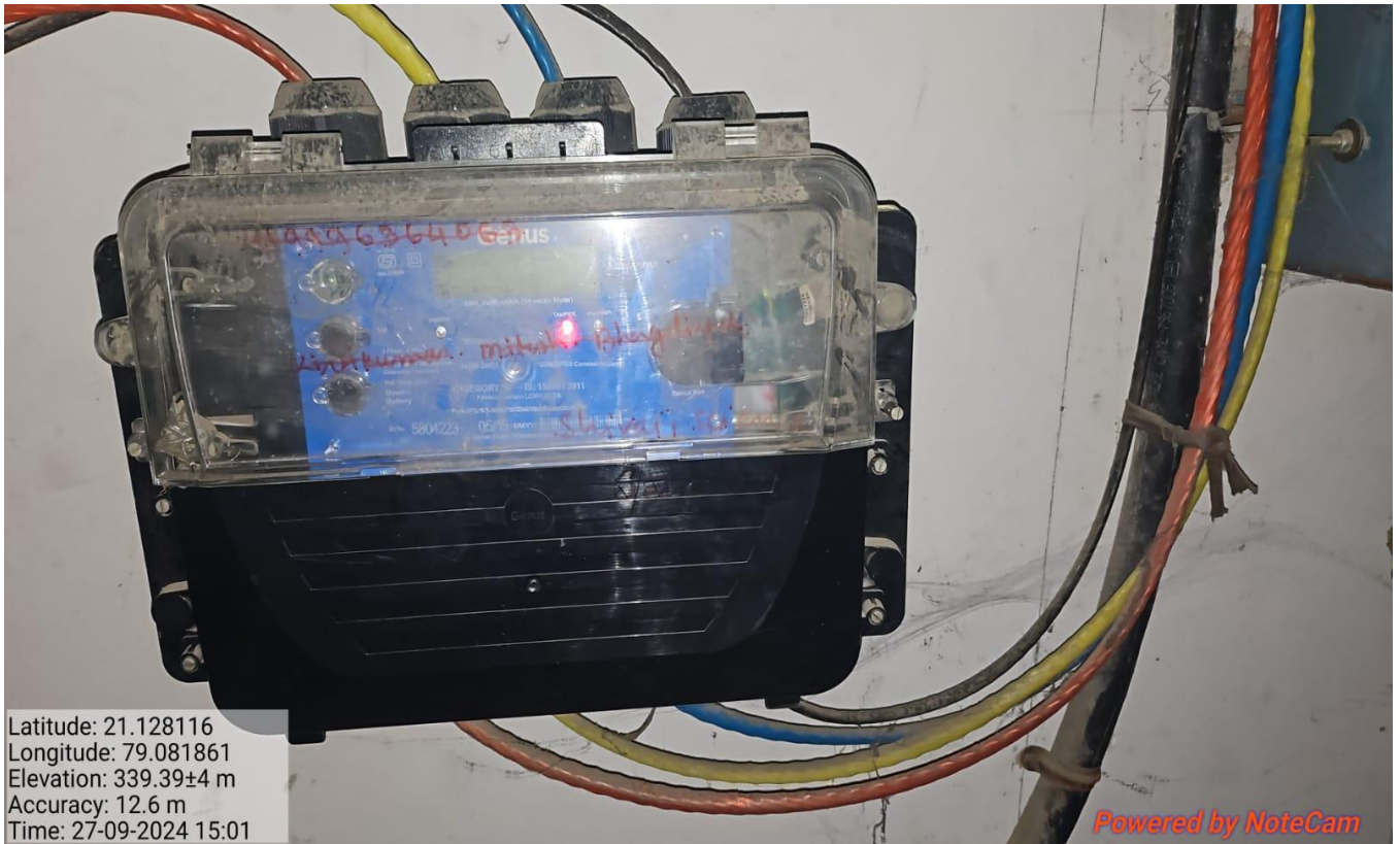
Solar panel meter of Block B
