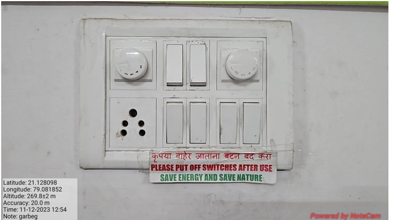
Signage for energy conservation
