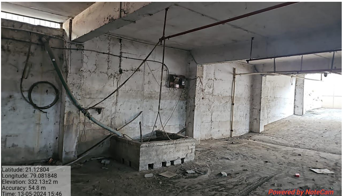
Chemicals from various department collected here in the separate tank and properly treated
