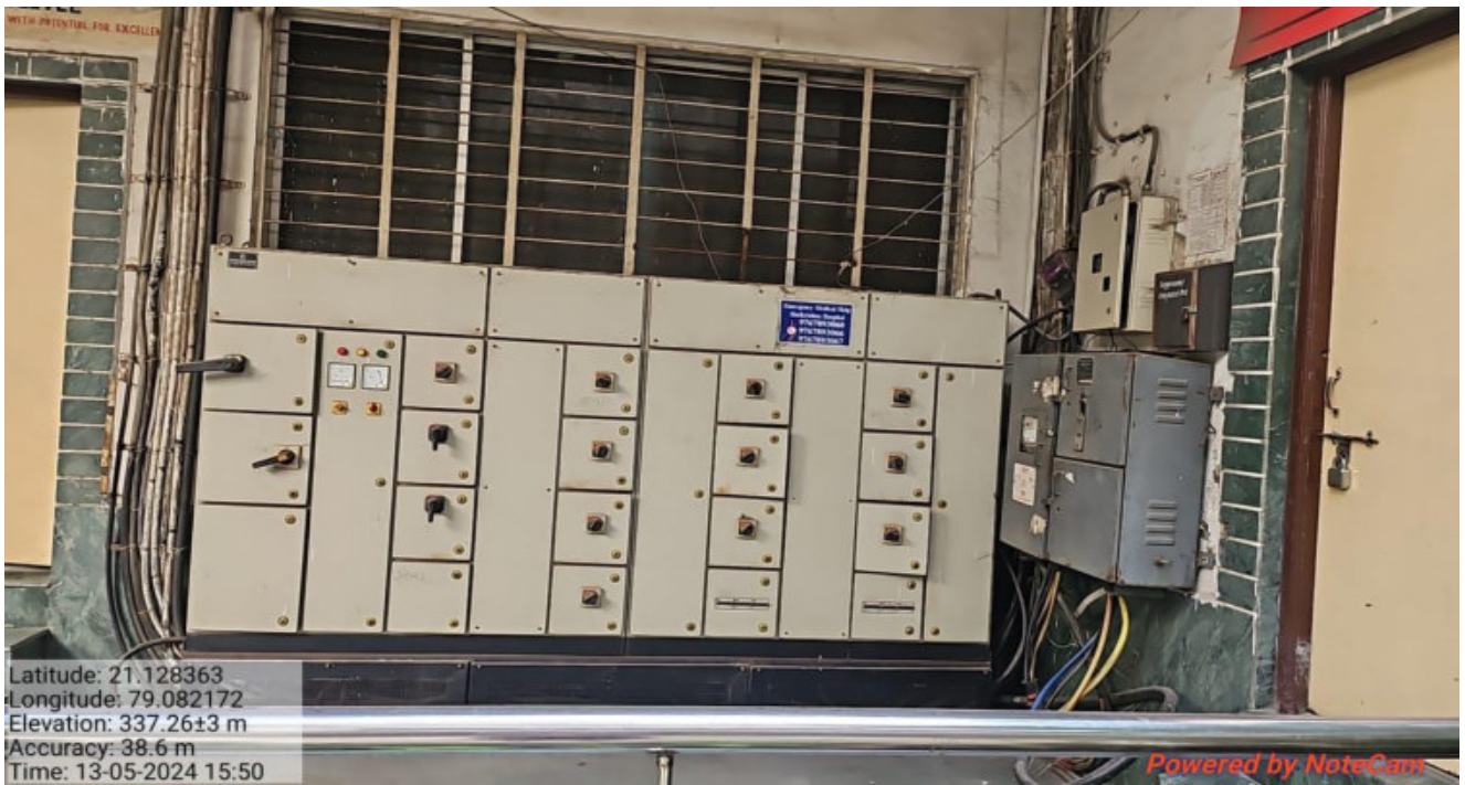
Solar converter / Generator /Electric distribution unit
