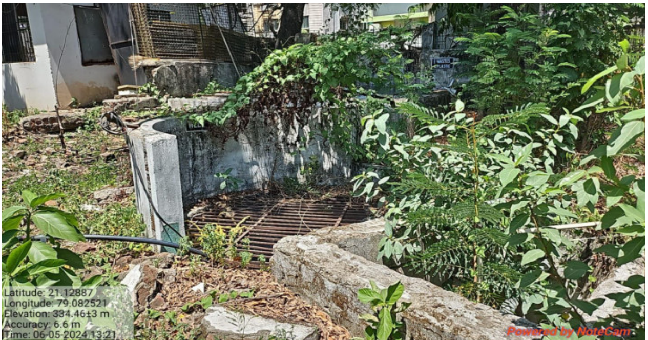
Bore well/ open well recharge
