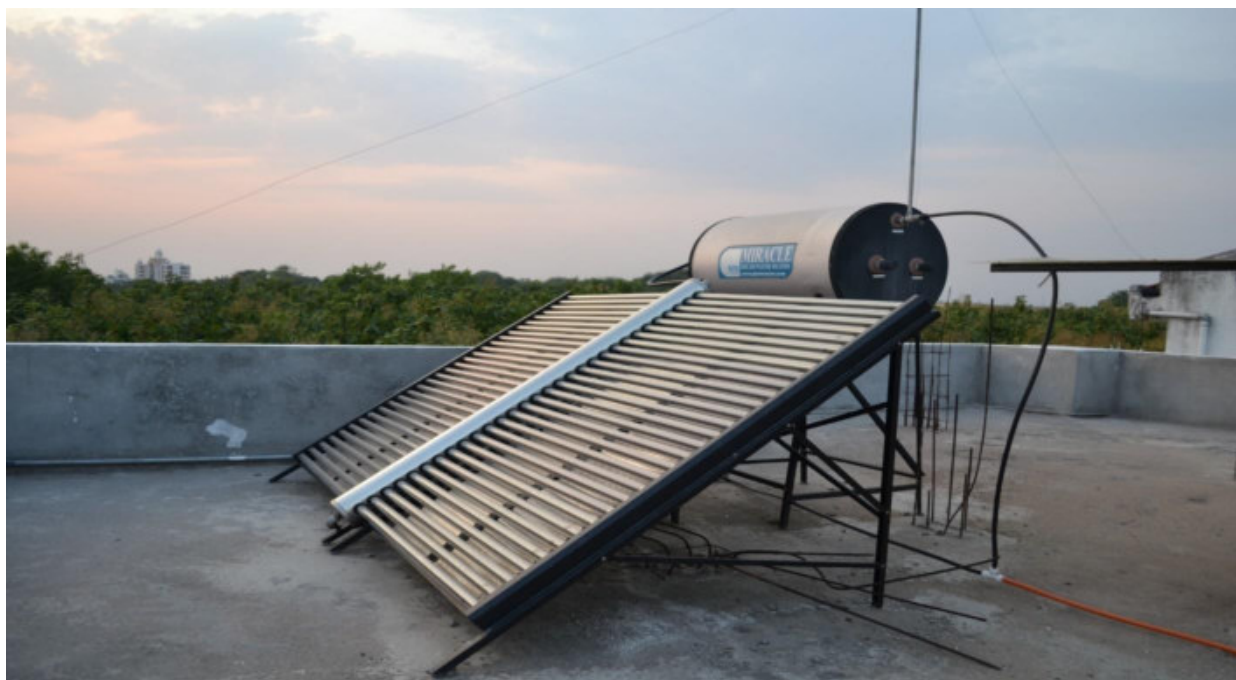
Solar Panel heater in Girls hostel
