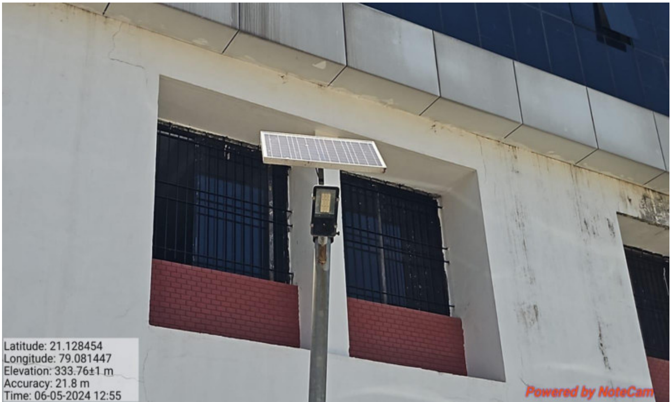
Sensor based energy conservation (Solar panel in ground)
