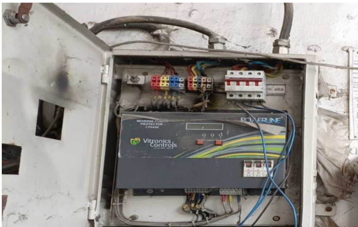
Solar converter / Generator /Electric distribution unit
