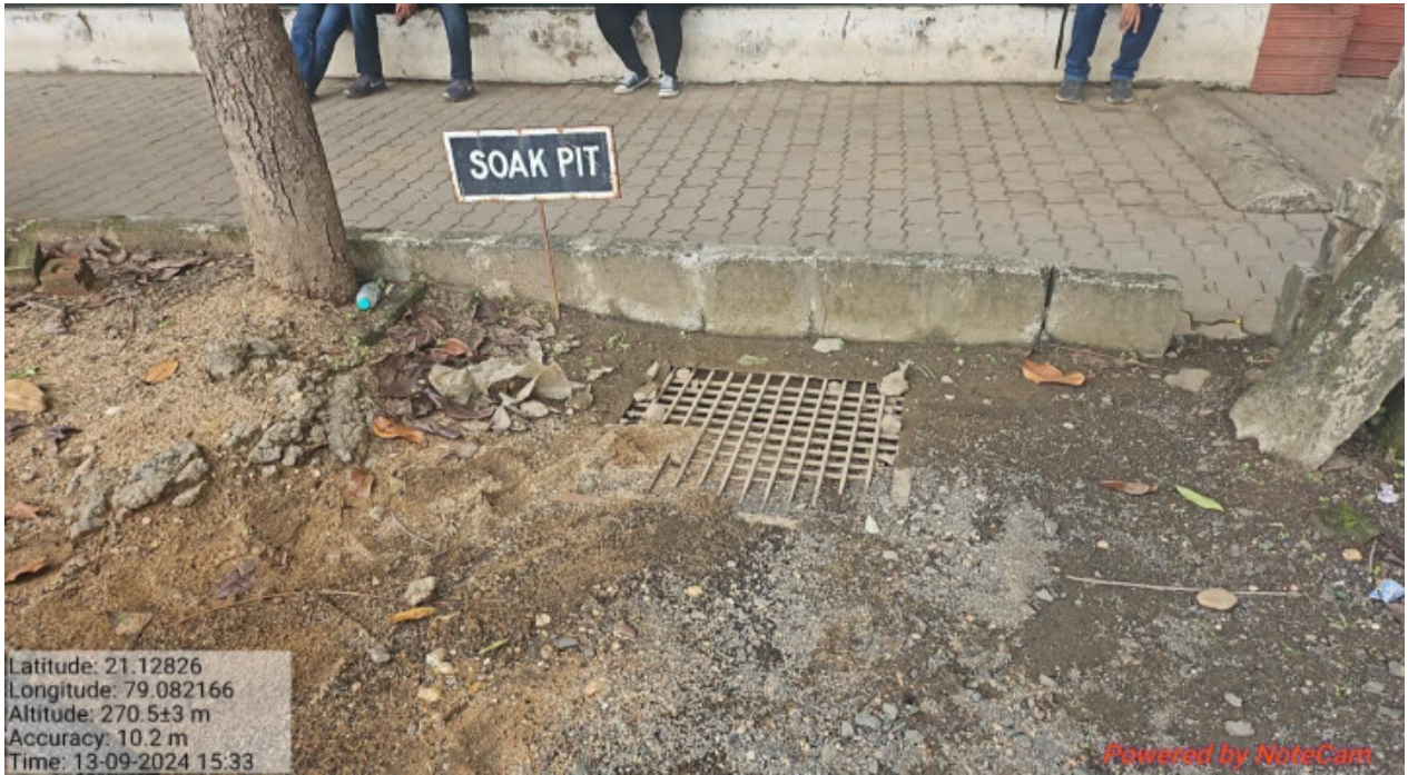
Rain water harvesting: Soak pit
